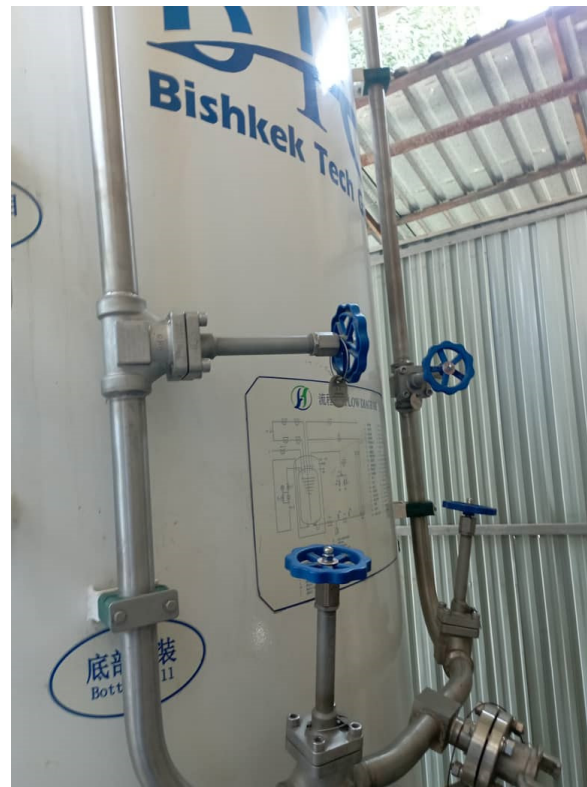
Image 3. Tank for the liquid oxygen gasification process installed in the Infectious Disease Hospital in Osh
